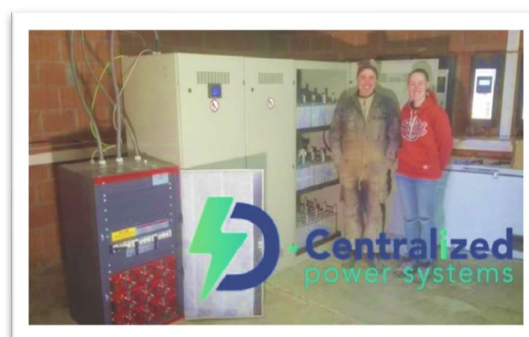
Greenergy 'Bigstorage' 60kW - 380Vdc – 215kWh 2020 (Gistel W-Vlaanderen)
